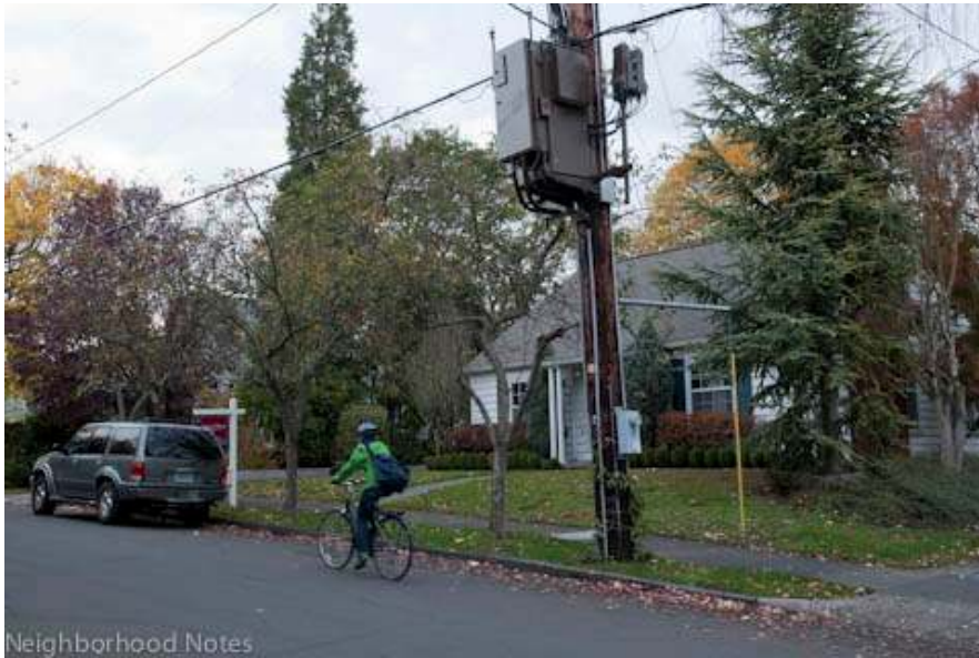
Some cell towers have equipment mounted to the pole.
