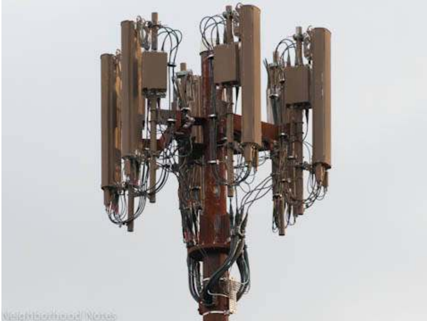
Cell towers contain multiple antennas.
