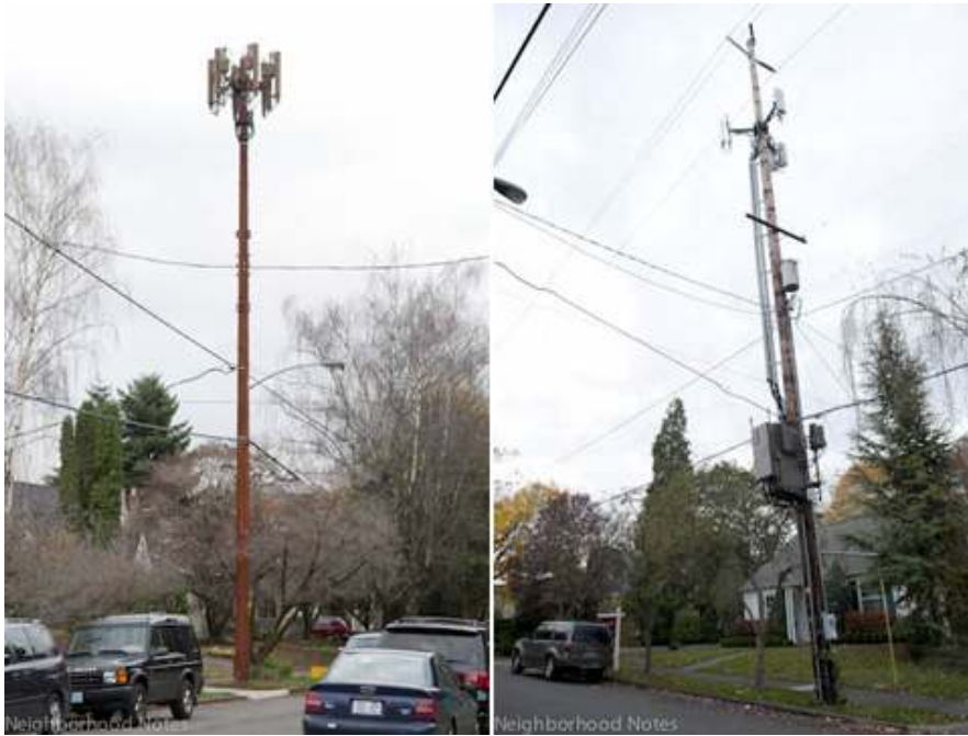
Cell towers can be varied in their height and appearance.
